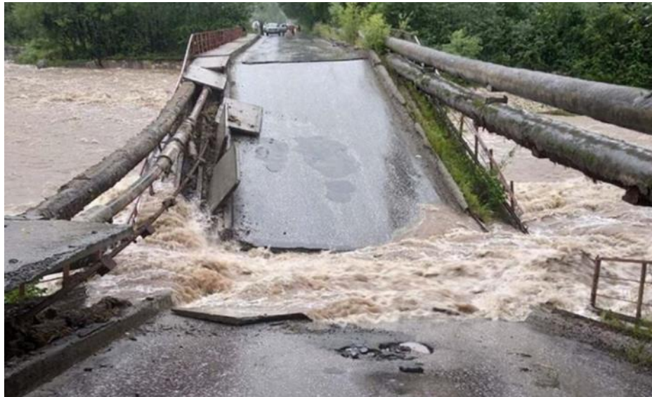
Fig. 1 Destruction of the bridge due to erosion of the riverbed under the bridge.
