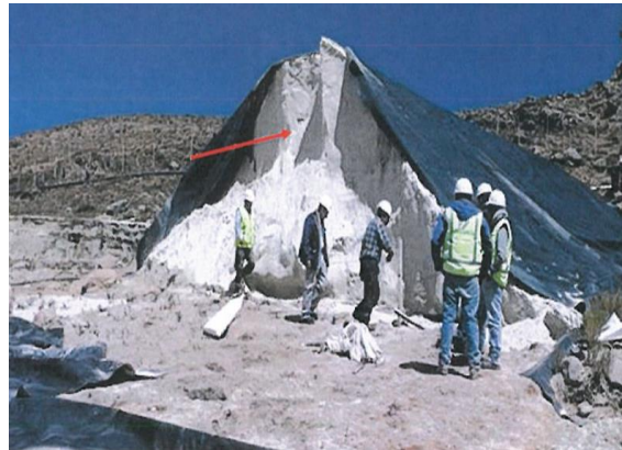
Figure 9. View of the breach of the tailings deposit No. 4 dam, with an almost vertical slope.
