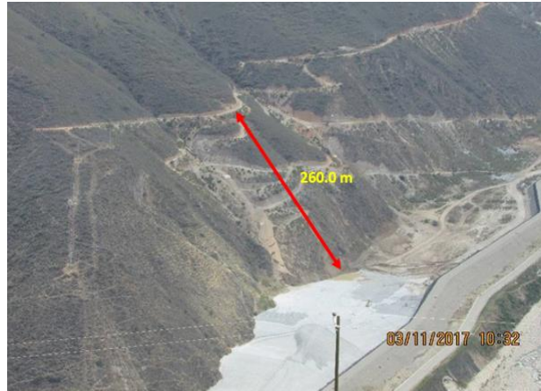
Figure 8. View of the distance between the crown channel and the Yuracyacu filtered tailings deposit, with drainage of uncontrolled runoff water in said section.
