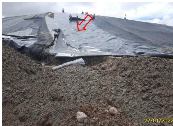
Figure 3. Gap covered with geomembrane after carrying out temporary repair on the main slope - northern area of the Huaybillo tailings deposit.
