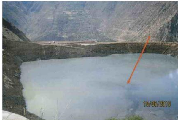
Figure 5. View of the water mirror in contact with the dam in the North Area tailings deposit.
